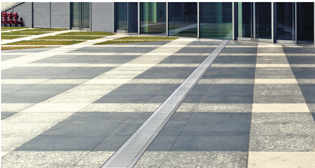
OFFICE PLAZA Product: T1500 (4") with Load Class C Stainless Steel Slotted Grates
